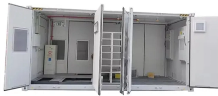
1075KW HH ESS
